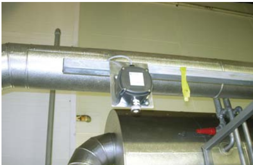
Refrigerant leak detector in a compressor plant room
