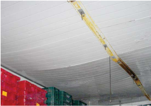
Damaged ceiling in a -18°C cold store
