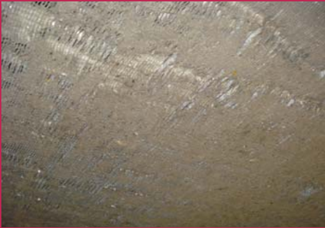
Build-up of debris on a condenser.
