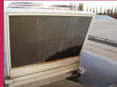
Oil stains on a condenser coil indicating a refrigerant leak
